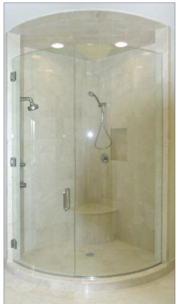
Custom Curved Enclosure
